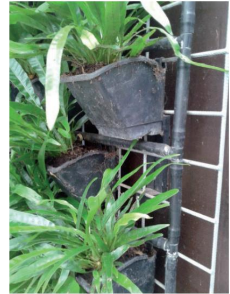
Fig. 8 Irrigation pipeline is provided on every level
